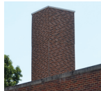
Faux chimney conceals 15 panel antennas
